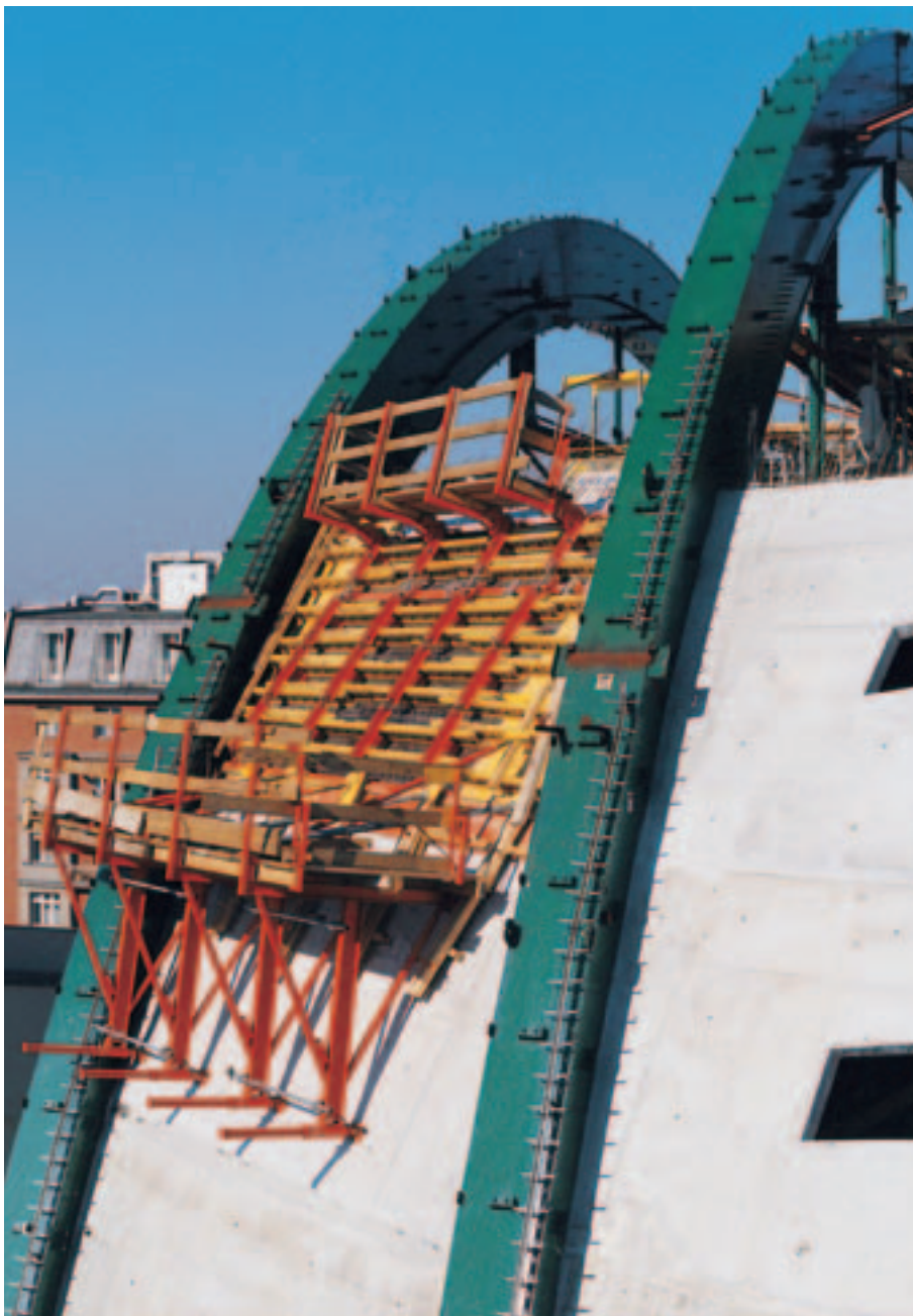
“Horizontally” positioned RUNDFLEX for the forming of an arched slab for a culture centre in Berlin.
