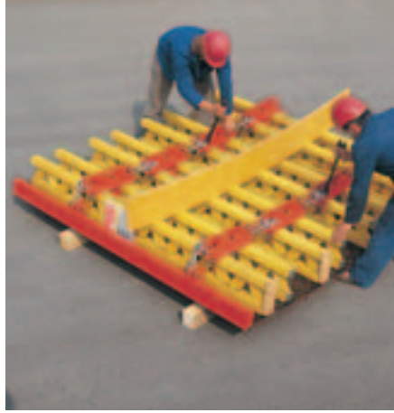
Checking the required curvatures is carried out by placing the radius template on the formwork girders.
