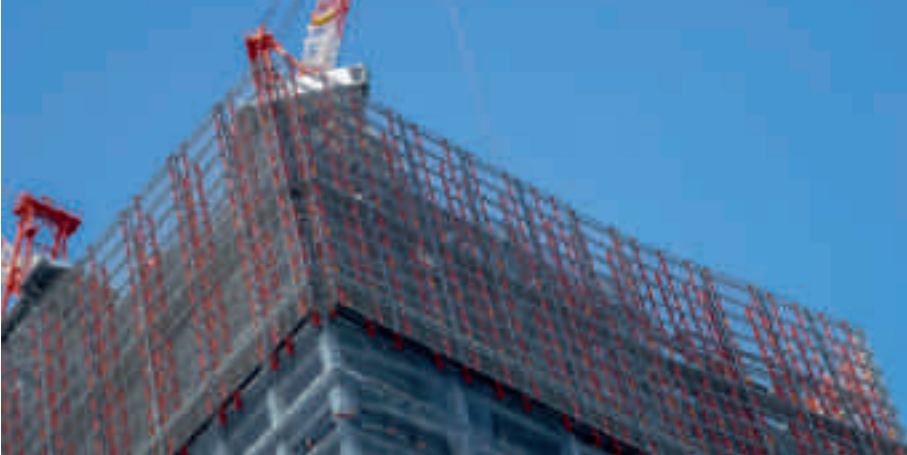
This gap-free mesh enclosure in Japan ensured a high level of safety while simultaneously providing light and air permeability.
