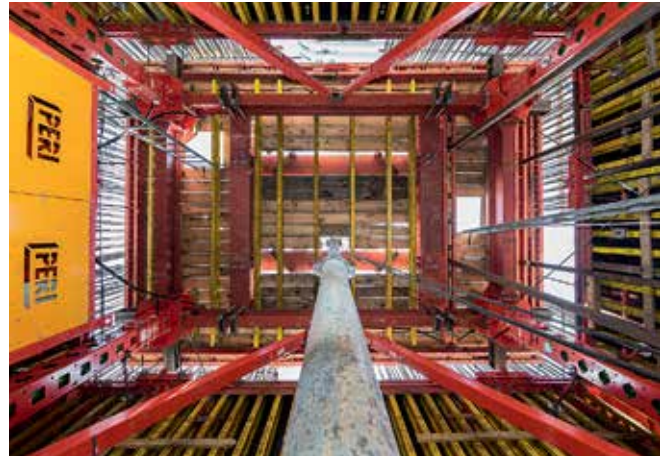
The ACS Core 400 ensured that the construction team was able to meet the extremely tight schedule.
